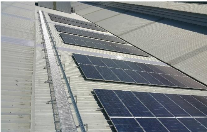
Thai Gow Gai (TGG) 561 kWp #Pathumthani
