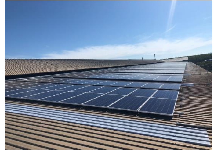
Mitr Steel 998 kWp #Rayong
